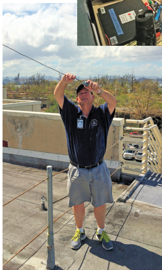
Gary Sessums, KC5QCN, installing a dipole antenna at the emergency operations center located at the Puerto Rico Convention Center.
